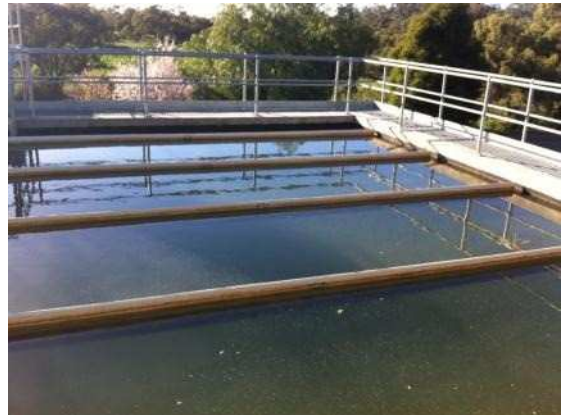
Figure 3-4: Sedimentation Tank at Hay WTP
